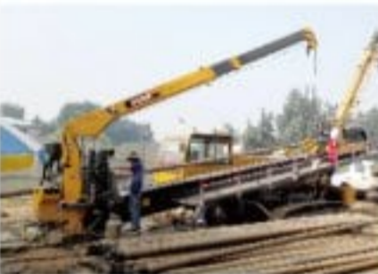
XZ3600水平定向钻机在山东泰安施工 XZ3600 HDD working in Taian Shandong
